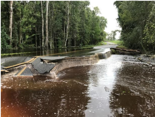
Roadway damage cause by erosion due to flooding during Hurricane Irma, 2017 – Bradford County File Photo
